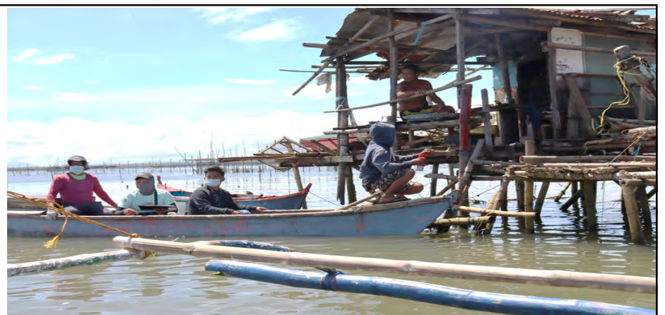
Marking team sprays red paint on a bamboo hut installed within Cavite waters to mark the same as one of the structures for demolition. Such bamboo huts serve as the houses of the caretakers of illegal fishery structures in the area---p.2
