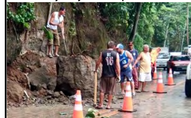
The picture shown a huge slab of a rock collapsed in Indang - Alfonso Road last August 12, 2018 which caused a hassle for some motorists from which authorities and residents had been helping to remove the rock slab. The incident occurred at the height of Habagat, which occurred after a few days of rain. The Indang - Alfonso Road is an all-inclusive national highway connecting the towns of Indang and Alfonso in the province of Cavite. Photo by Reyland Lopez
